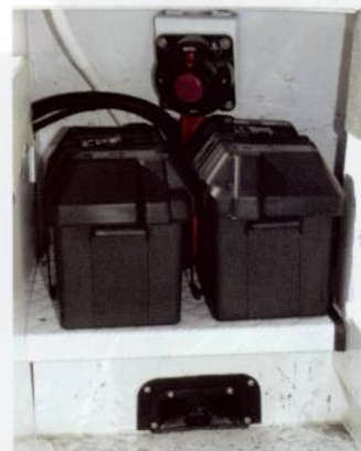
Batteries sit up off the floor and offer easy access to the battery switch.
